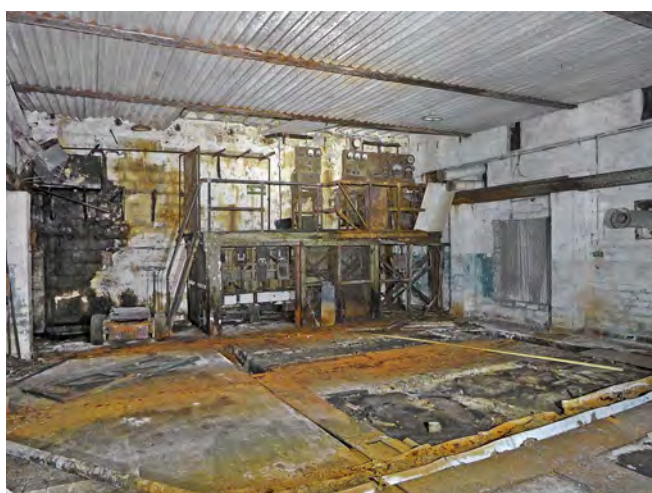
Hay's Level: A more substantial chamber which appears to have contained large generators
